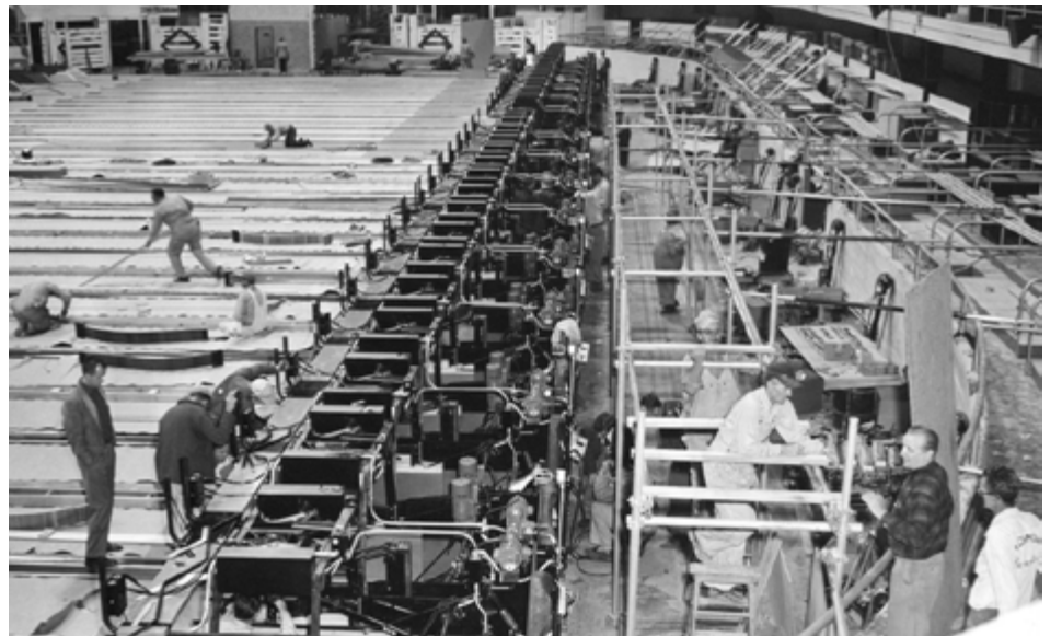
AMF lanes, machines (the automatics!) and under lane ball returns being installed at the 1957 USBC National Championships in Fort Worth, Texas (Credit: USBC Open Championships)
